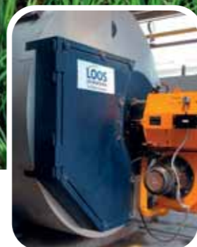
Gas Fired Steam Boiler
